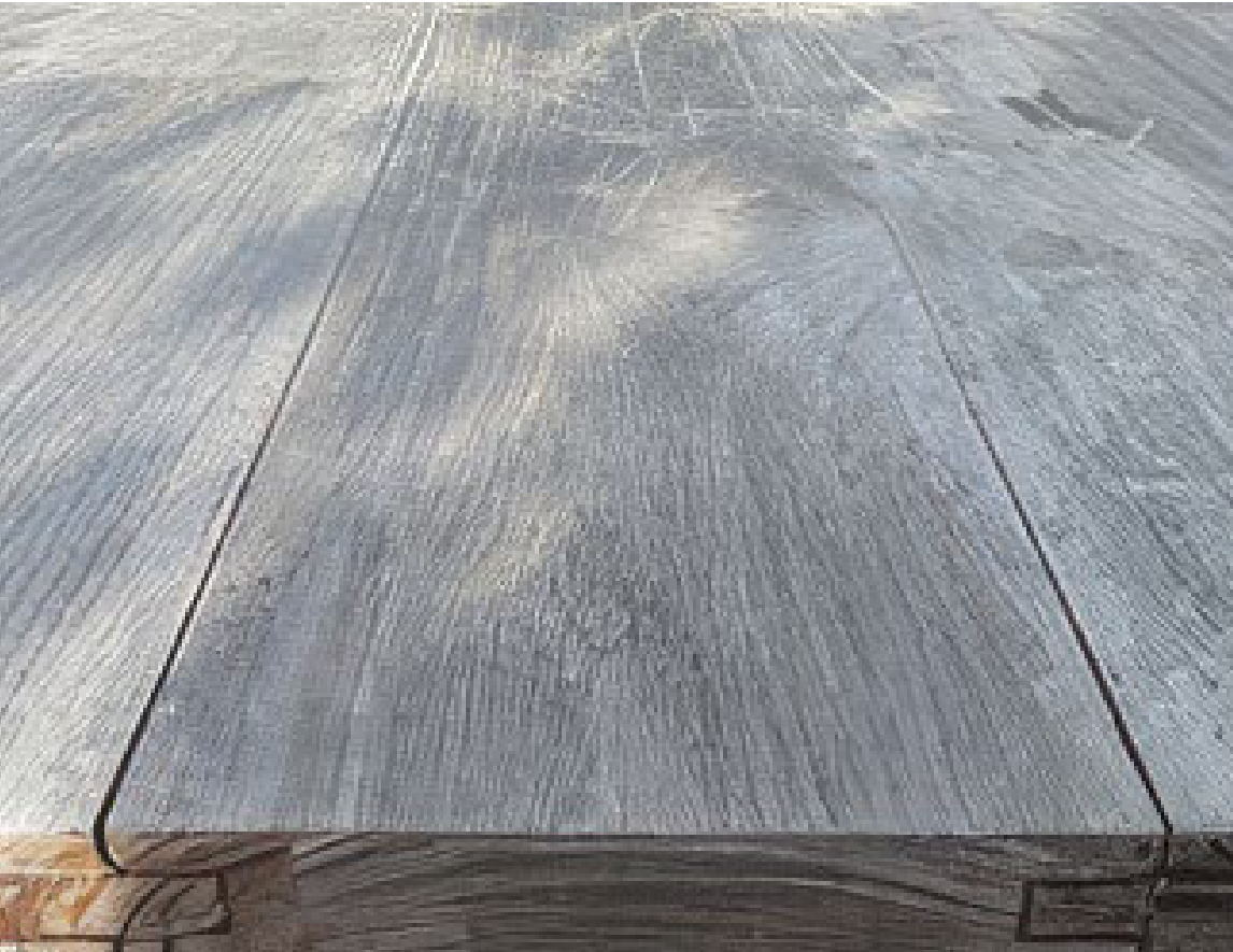
Example of sun-degraded wood.
